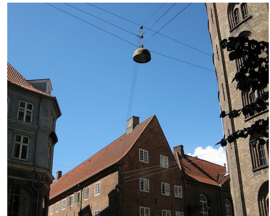
Catenary lighting Copenhagen, Denmark.
