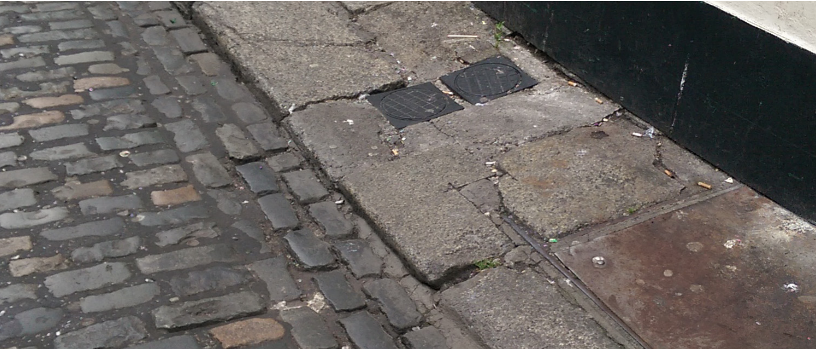
Granite pavement flags in poor state of disrepair
