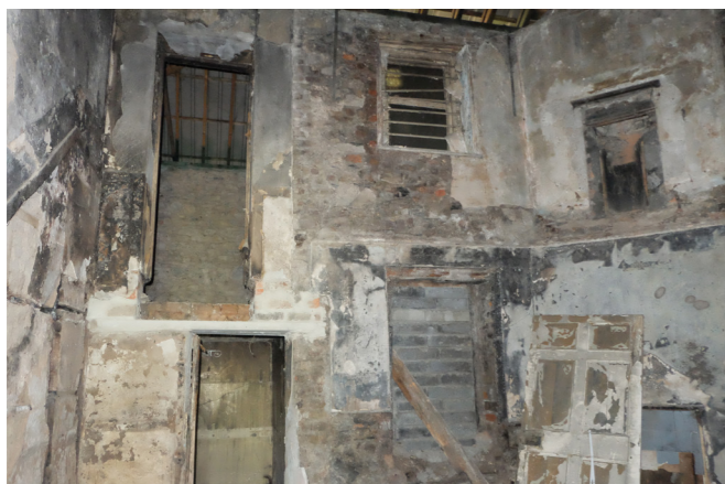
Fig. 2.15 The interior of the central, 18th century wing. All the upper floor structure has been lost, but fireplaces and a two storey partition survive.
