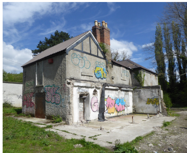
Fig. 2.14 The house from the south west: 18th century wings, with 19th century wing behind. Scars of demolished single storey 20th century extension in foreground.
