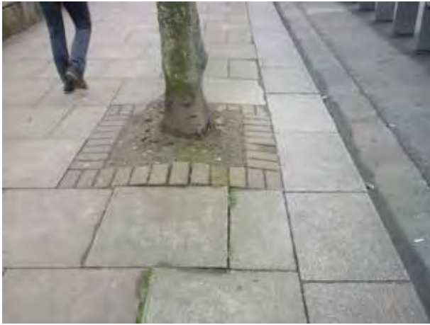
Fig. 64 Detail of paving being disturbed by tree in footpath.
