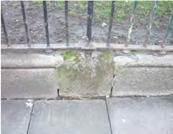
Fig. 36 View of granite plinth damaged by rusting pale.
