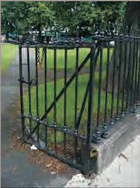
Sandymount Green is bounded by simple wrought and cast-iron railings with a curved railing to the corners. Inset shows one of the gated entrances.
