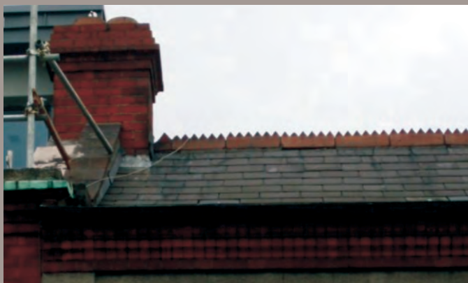
Original natural slates and terracotta ridge comb on Sandymount Road. Note the stepped brickwork to the gutter.
