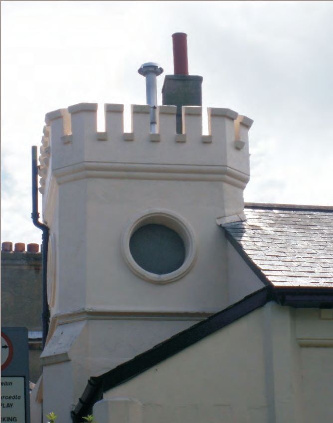
Roof details showing square profile tower with battlements, chamfered corners and circular window openings.
