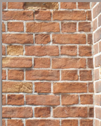
Mid nineteenth century fired red brick on Gilford Avenue showing some spalling in places
