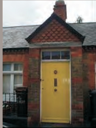
Late nineteenth century entrance porch with tongued and grooved door. The fish scale terra cotta tiles above are an attractive feature.
