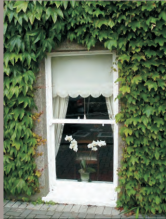
Single pane sash window with convex horns with ring pulls on the sashes.
