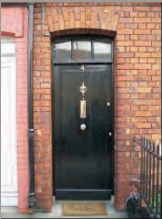
Tongued and grooved timber door with glazing bars to the original overhead.
