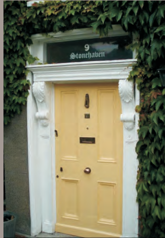
Nineteenth century flat panelled door with overlight supported on carved timber corbels and flat panelled pilasters. The overlight is an unusual feature, as this period of entrance door would more typically have a fanlight.
