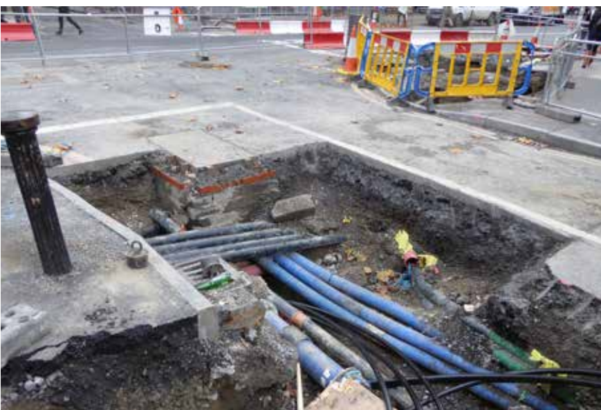
Congestion of underground services poses a challenge to urban tree planting and in particular, tree roots. Photo by Marc Coyle.
