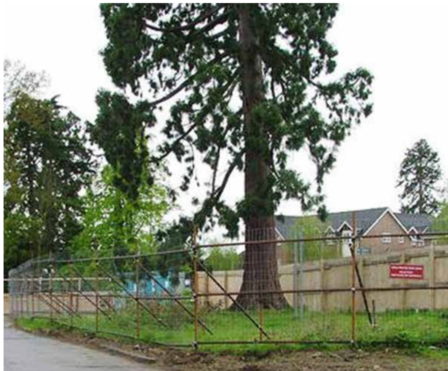
Adequate fencing prior to commencement of construction works is essential to prevent damage to the root zone of retained trees.
