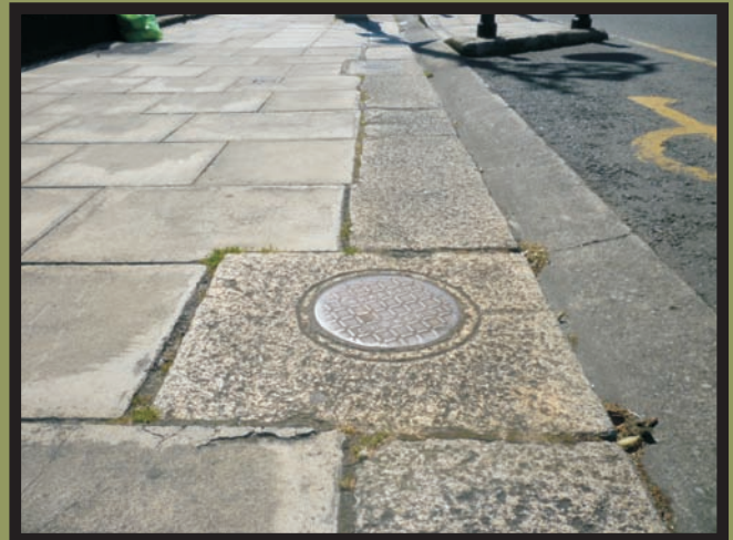
Figure 23 : Coal hole cover.
