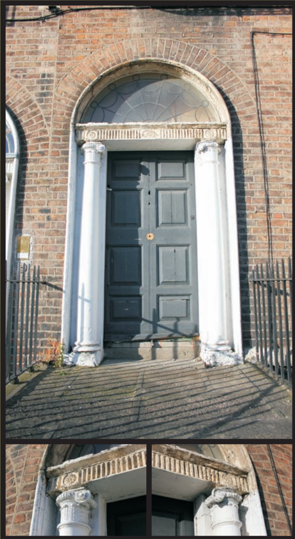
Figure 9: No. 15 Typical panelled door in timber door surround, with intricately detailed fanlight (without side lights)
