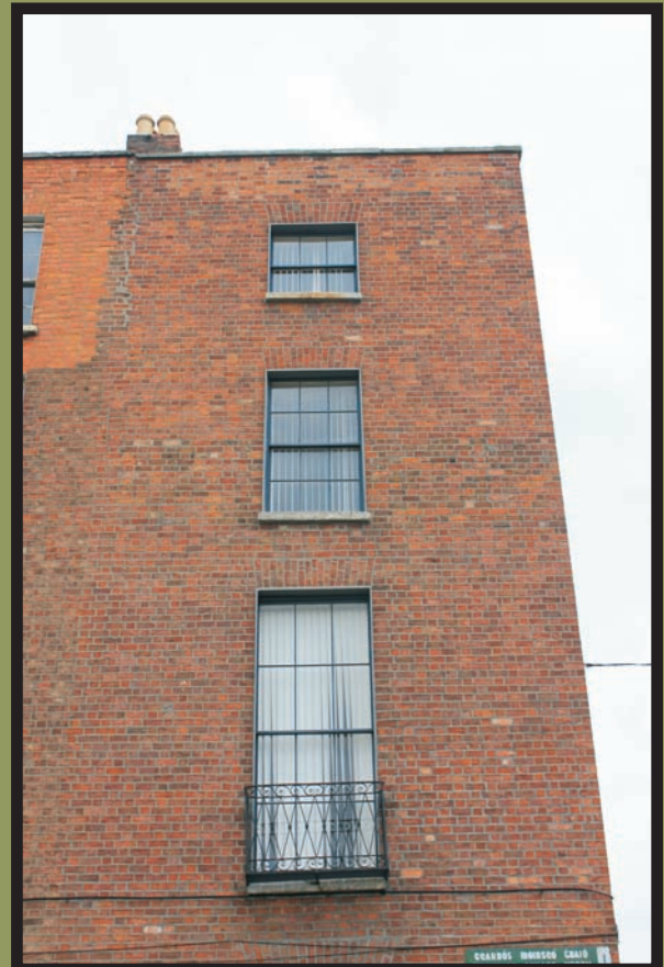
Figure 8: Typical hierarchy of sash windows to Georgian townhouse, with 6-over-6 sashes to first and second floors and 3-over-3 sashes above
