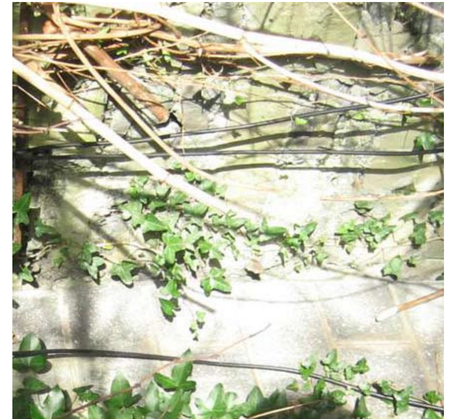
Detail view from east side, showing stones to tunnel entrance arch. Opening is filled with concrete block.
