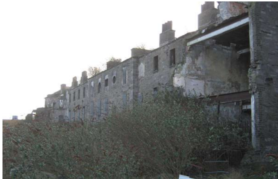
North elevation of surviving southern wing—showing the truncated western return wing of the original quadrangle complex. This photograph also illustrates the poor condition of this structure.
