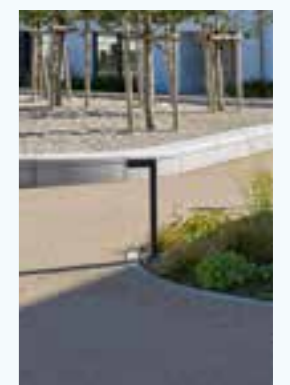
Lighting bollard at edge of planting bed
