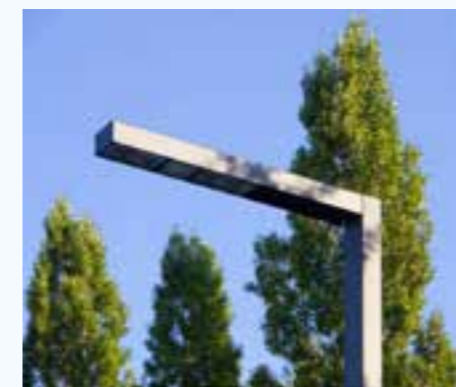
Example of column mounted luminaire
