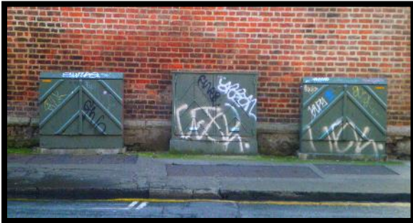
Figure 65 - Corner of North Great Georges Street and Denmark Street Great - prominent junction boxes representing opportunity for innovative street art
