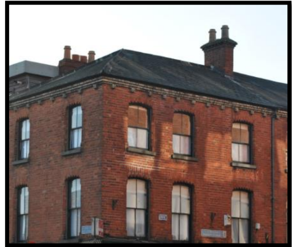
Fig 54 – No. 14 Denmark Street Great - 19th Century roofscape with hipped end roof and brick chimney stack with pots
