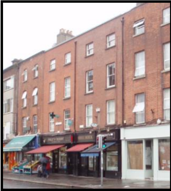
Figure 49 – No. 134 Parnell Street Inappropriate replacement upvc or aluminium top hung windows at upper floor levels – breaking the vertical rhythm of the 19th Century streetscape
