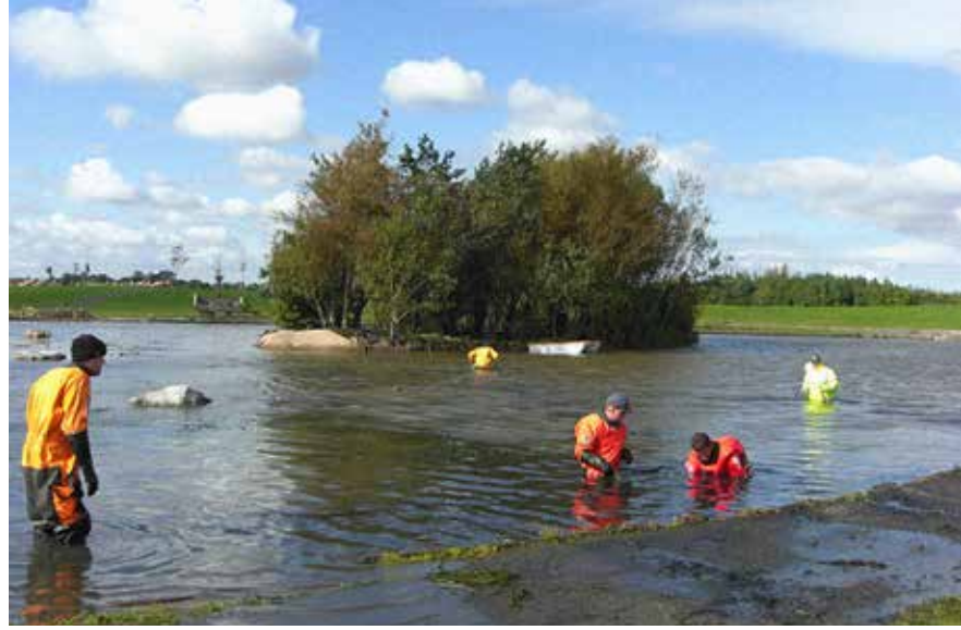
Preparing the pond by clearing debris prior to installation of matting (Photo: Maryann Harris).
