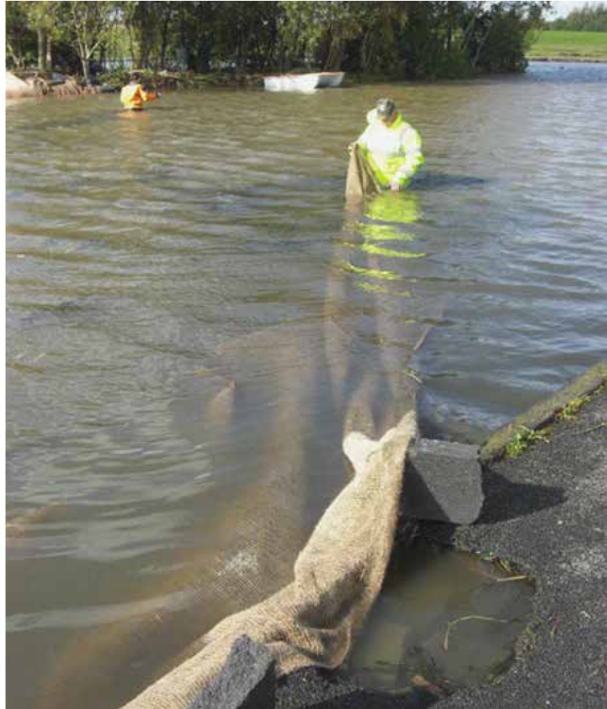
Laying jute matting at the pond at Darndale Park to control Curly Waterweed (Photo: Maryann Harris).
