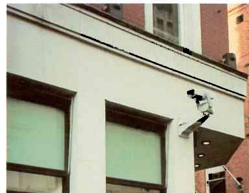
▼ Discreetly mounted CCTV cameras provide a visually acceptable security system for larger stores.
