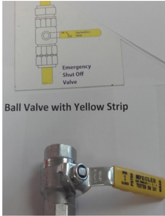
Photograph 6: Ball valves with yellow strip after regulator and before appliance (2 per run serving an appliance)
