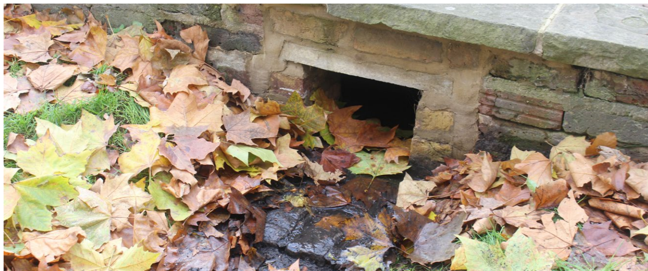
Polluted silts collecting from a busy road at an inlet apron allows for easy removal
