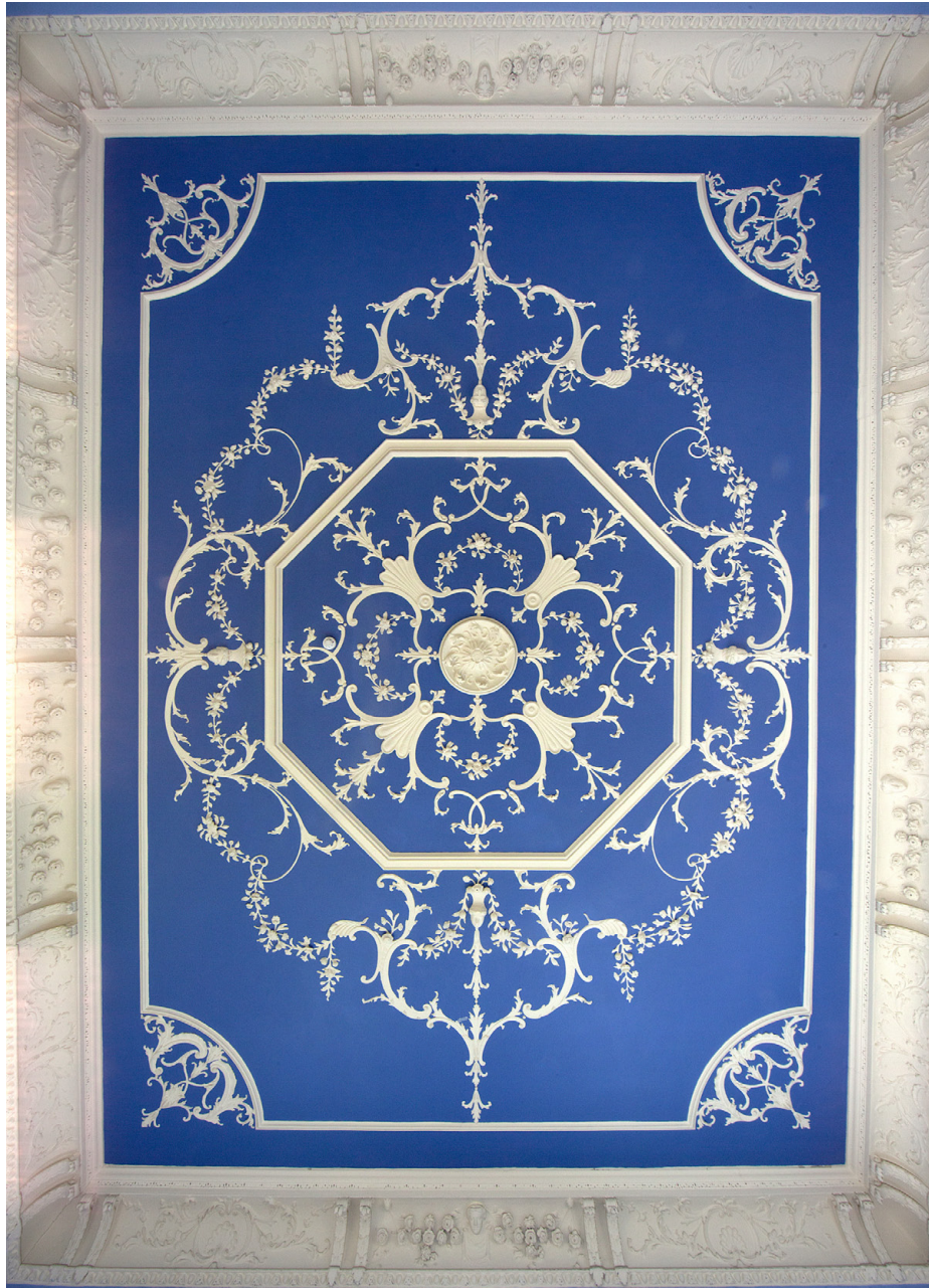
No. 4 Parnell Square, first floor front room ceiling. Photo: Paul Tierney Photography
