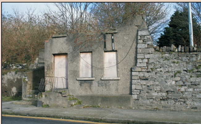
Derelict house, Gamble's Buildings, Main Street
