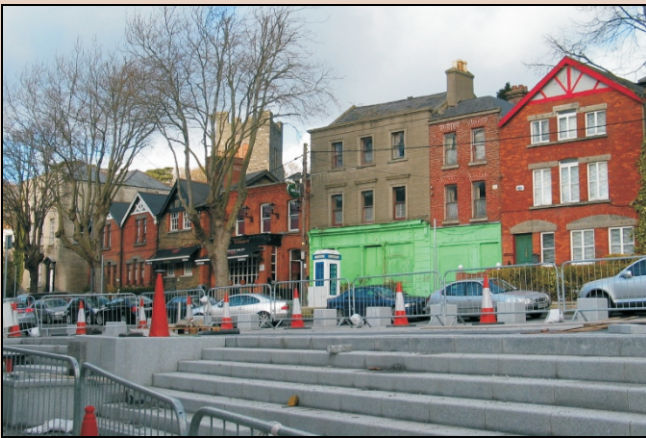
View from west side of newly refurbished square to east side of Martin's Row.
