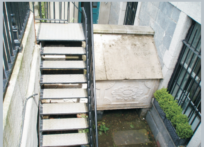
Photo 2.1.1.2 No. 3's front basement area retains its granite flagstones and an original watertank.
