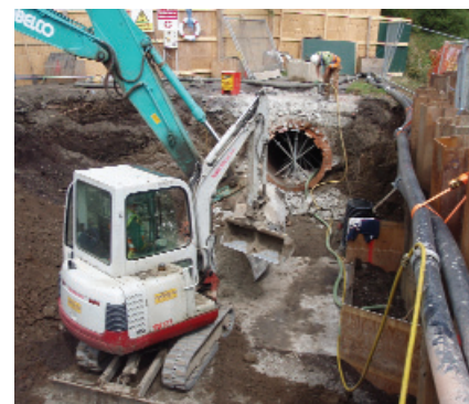
Rathmines & Pembroke Trunk Sewer being diverted along Dodder river (as part of Aviva Stadium Works)
