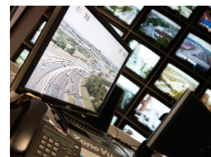
Traffic Control Centre
