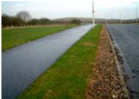
Roadside filter drain.
