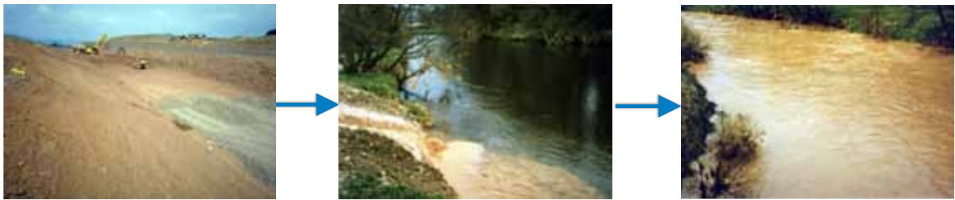
M74 construction led to pollution of the River Annan which spread rapidly.
