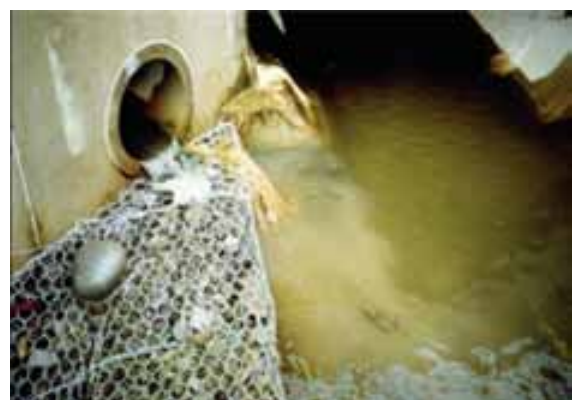
Polluting discharge from filter drain, M74.
