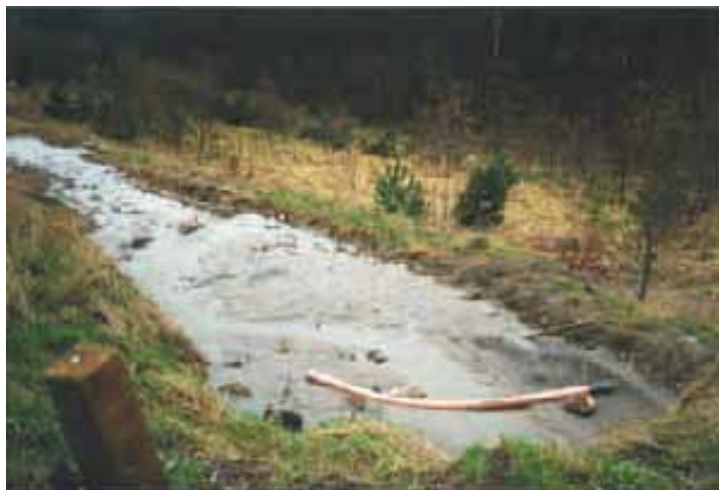
Figure 53: An Example of Damage Caused by Routing Construction Runoff through a Permanent Swale
