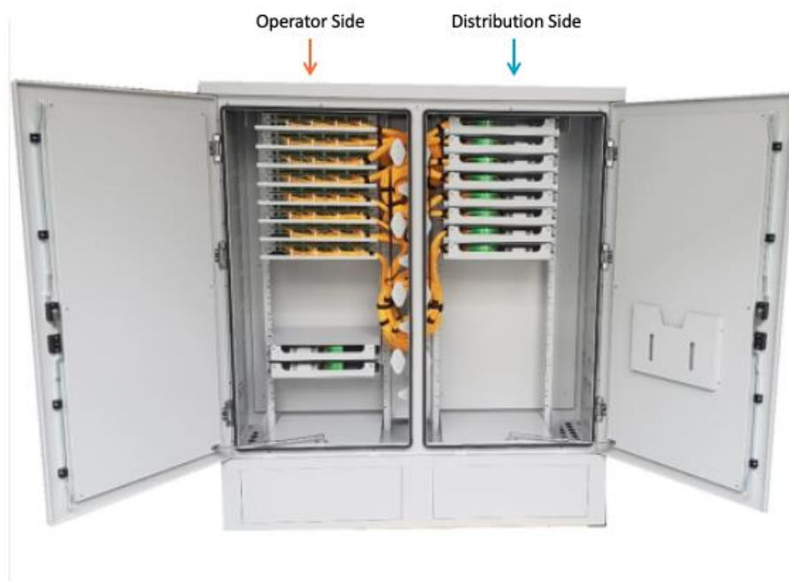
Fig 5. Typical example of a multi-Service Provider PDP patch panel.
