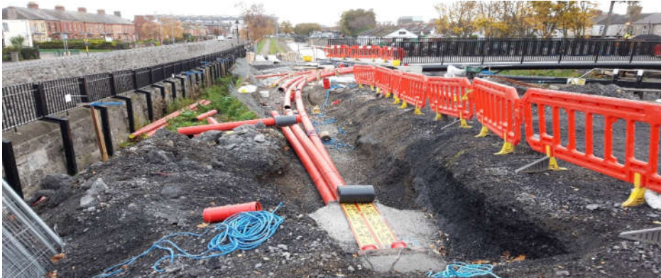
Duct installations on north side towpath
