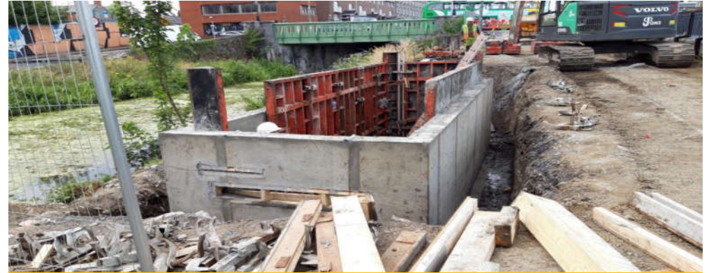
ESB HV joint bay near Cross Guns Bridge
