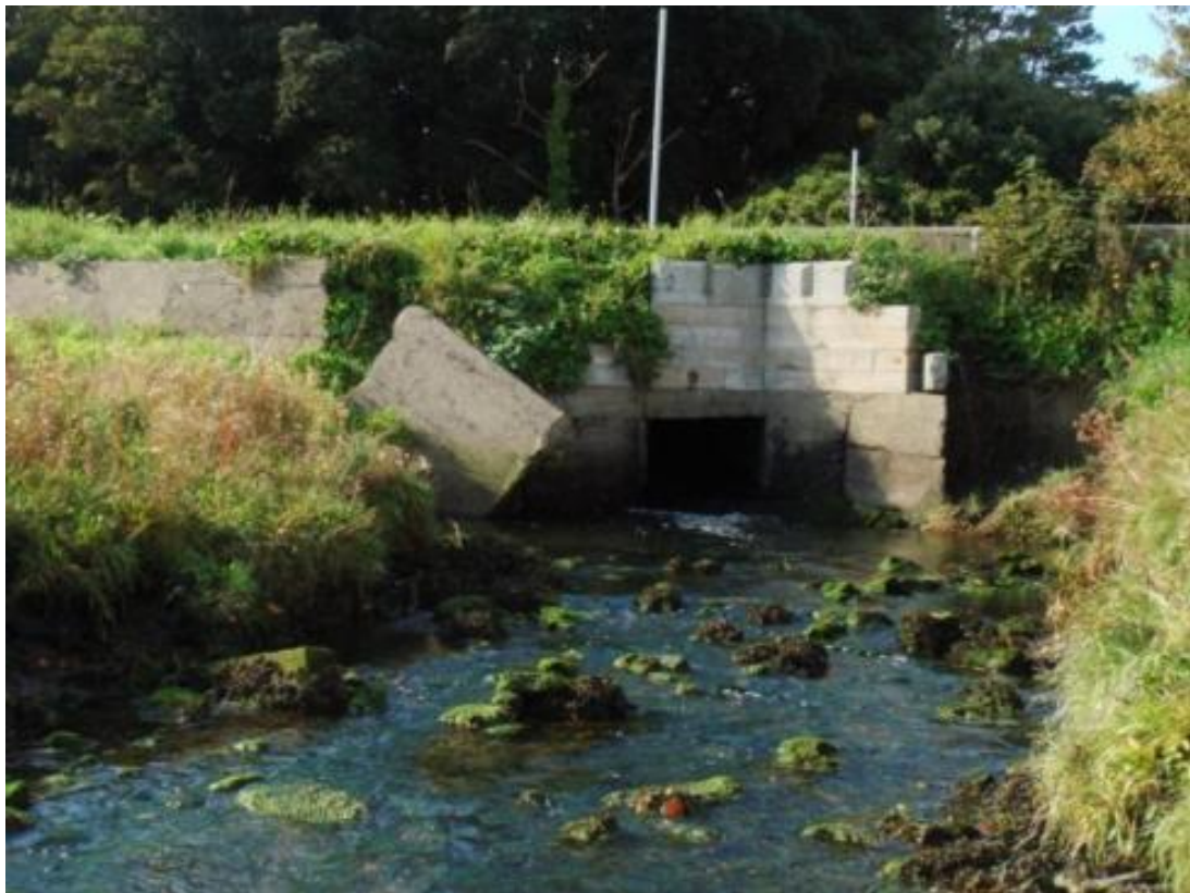
Photo 4.1 Collapsed section of wall at Naniken Stream culvert
