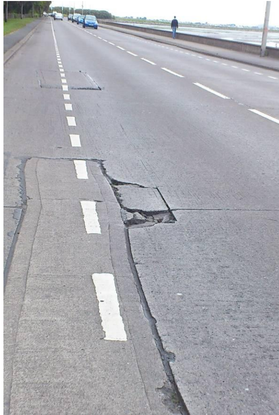
Photo 3.1 Condition of Existing Road Pavement on James Larkin Road
