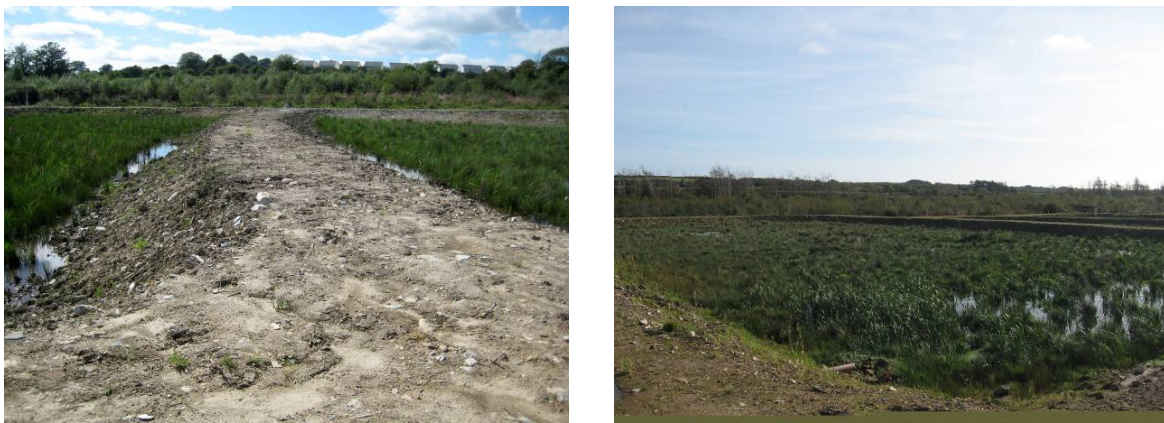
Figure 1 ICW two months after commissioning
