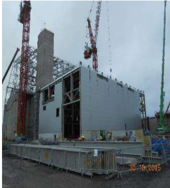
Turbine Hall (Copyright PML).
