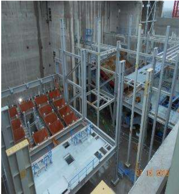
Boiler Hall (Copyright PML)
