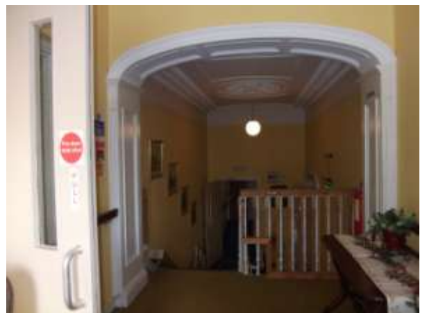
View of panelled timber linings to segmental headed arched opening to main staircase at first floor landing
