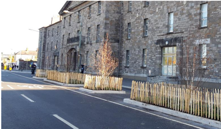
Resurfacing, road markings and construction of buildouts on Grangegorman Lower is complete. Installation of buff coloured pedestrian surface will be completed in the coming weeks.
