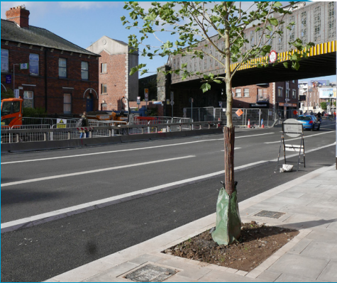
Bespoke designed tree pits are being installed to support new trees on the scheme
