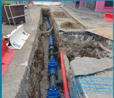
Approximately 6km of 100 year old watermains are being replaced throughout the route
