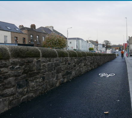
Reconstructed historic stone wall with cycle track open on North Strand Road
