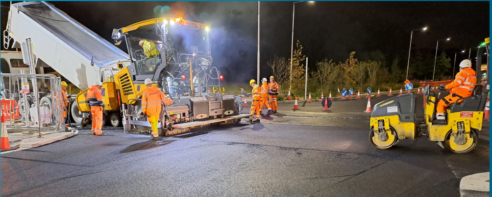
Road re-construction at each of the major junctions along the route continues
