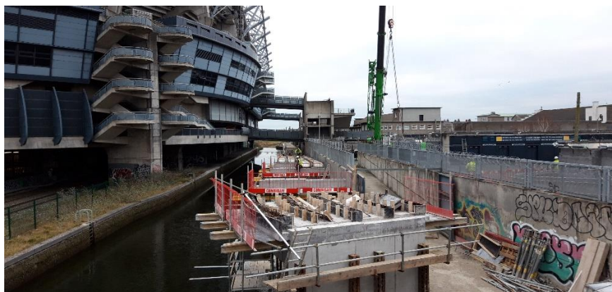
Precast ramp U- beams being lifted into place on east side of Bloody Sunday Bridge
