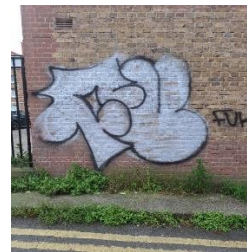
Graffiti removed from multiple locations in the complex by Housing Maintenance (before and after).
