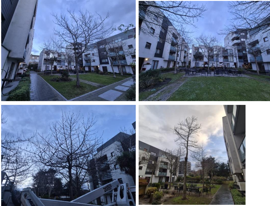
Tree removal and pruning carried out to maintain safety and clear access in the complex.
