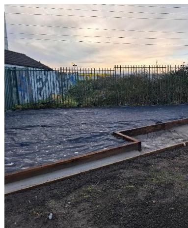
Cherry Orchard— raised bed area being prepared for raised bed and bench
