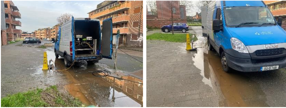
Graffiti removal and power washing have been carried out at Dolphin House.
