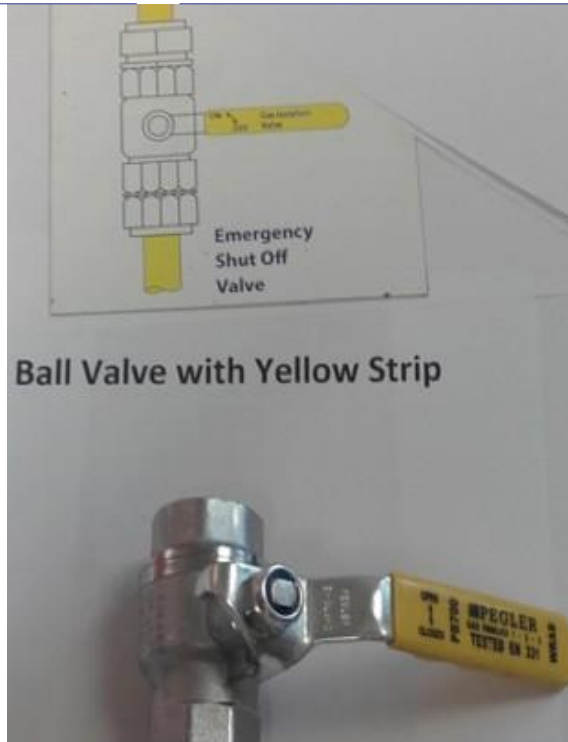
Photograph 6: Ball valves with yellow strip after regulator and before appliance (2 per run serving an appliance)
