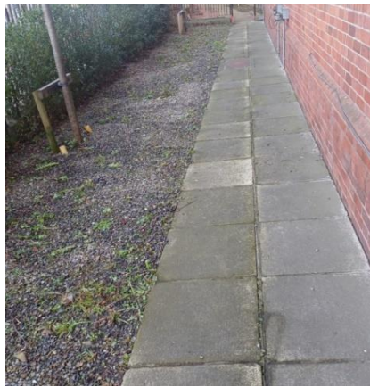
Weeding and removal of heavy vegetation along the complex's exterior perimeter. (before and after the works).
