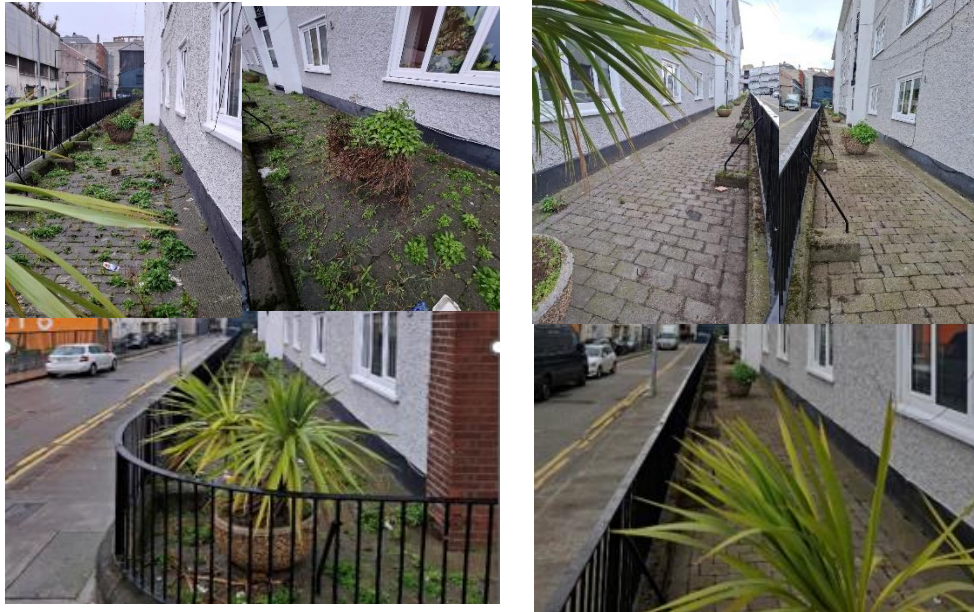
Clearing of weeds and overgrown vegetation along the exterior perimeter of the complex. (before and after the works).
