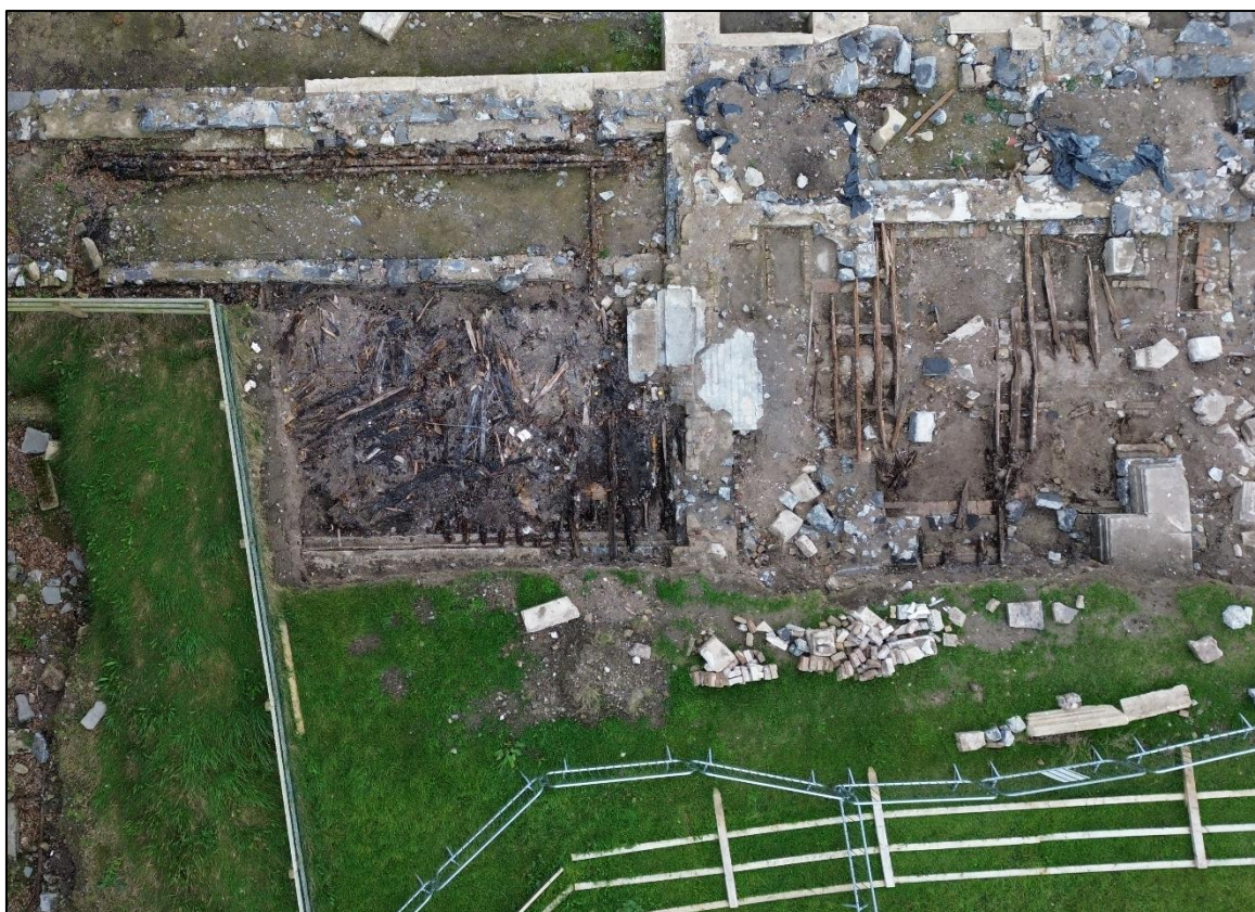
Plate 7 Aerial view showing the remains of charred timbers and off-centred fireplace setting in the picture gallery, to the right are the unburnt joists of the main hall
