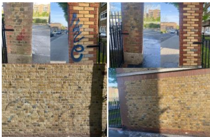
Removal of graffiti in the Oliver Bond House housing estate. (before and after).
