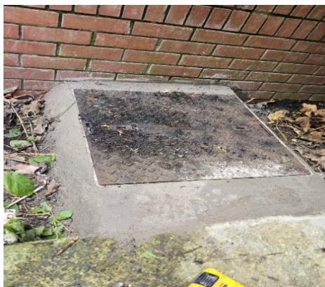
Drain access points with installed secure covers.
