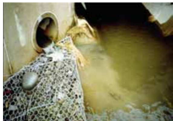
Polluting discharge from filter drain, M74.
