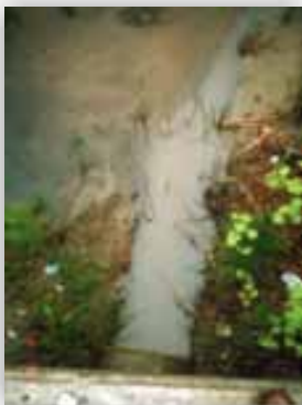
Effluent Discharge - Dry Weather Flow
